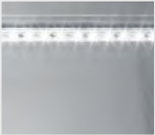
Illuminazione a LED LED lighting
